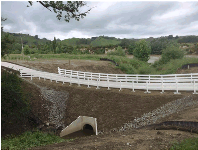
Photo: Section of new Mountains to Sea Shared Pathway just south of new bridge in Upokongaro
