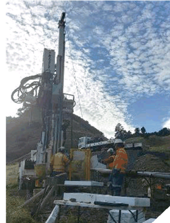
The crew at Te Oreore site drilling boreholes and installing groundwater monitoring devices, deep within the landslip area
